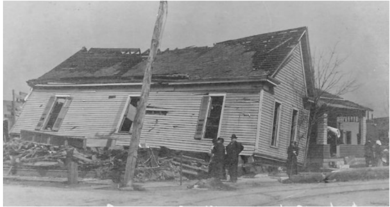
Charlestown Road and Vincennes Street took the blow hard
